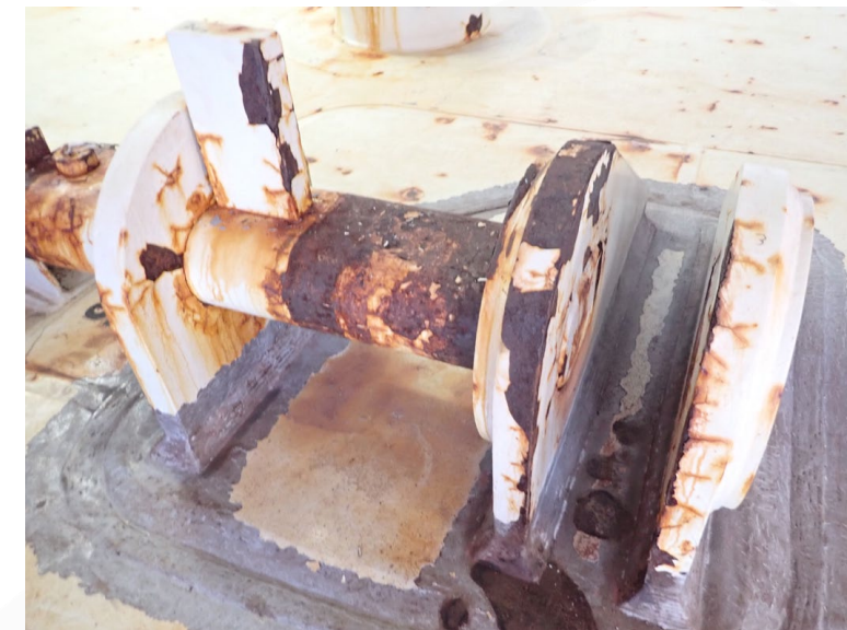
Corroded Smith Brackets. Function testing
